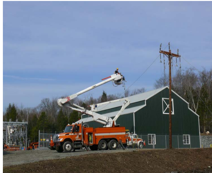
Housing Structure for Synchronous Condensers Winhall, VT
