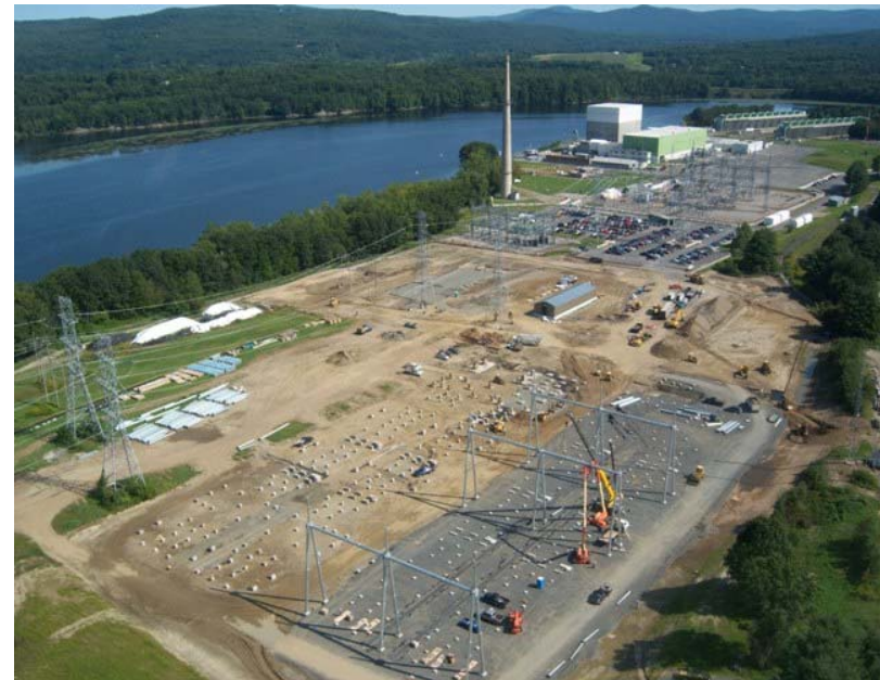
New 345kV Switch Yard Under Construction Adjacent to Vermont Yankee Nuclear Power Plant
